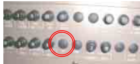
Figure 2-4 Circuit breaker location (Typical)
